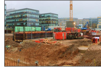
Start of construction work for new production and development centre in Cologne
